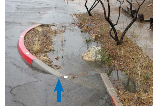
The concrete curb to the right of the blue arrow is flush with the street
