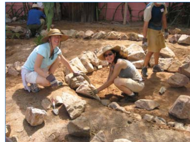
Volunteers pitch in to create bioretention basins at a ROW GI site in Tucson.
