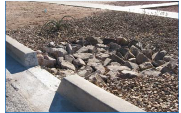
A rip-rap apron protects against soil erosion where curb cuts draw stormwater into bioretention areas.
