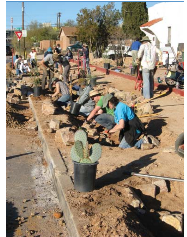
Volunteers install bioretention basins in the right-of-way at a workshop in Tucson led by Watershed Management Group.
