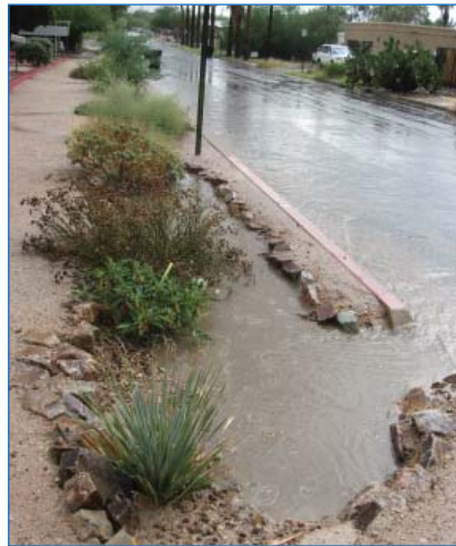
A curb cut draws stormwater from the street into a bioretention basin in the right-of-way.
