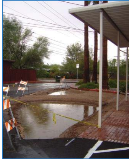
At this Tucson City Council Ward office, asphalt was removed from an unused portion of the parking lot. Runoff from the lot (foreground) and the adjacent building fills the unfinished basins in a summer storm.
