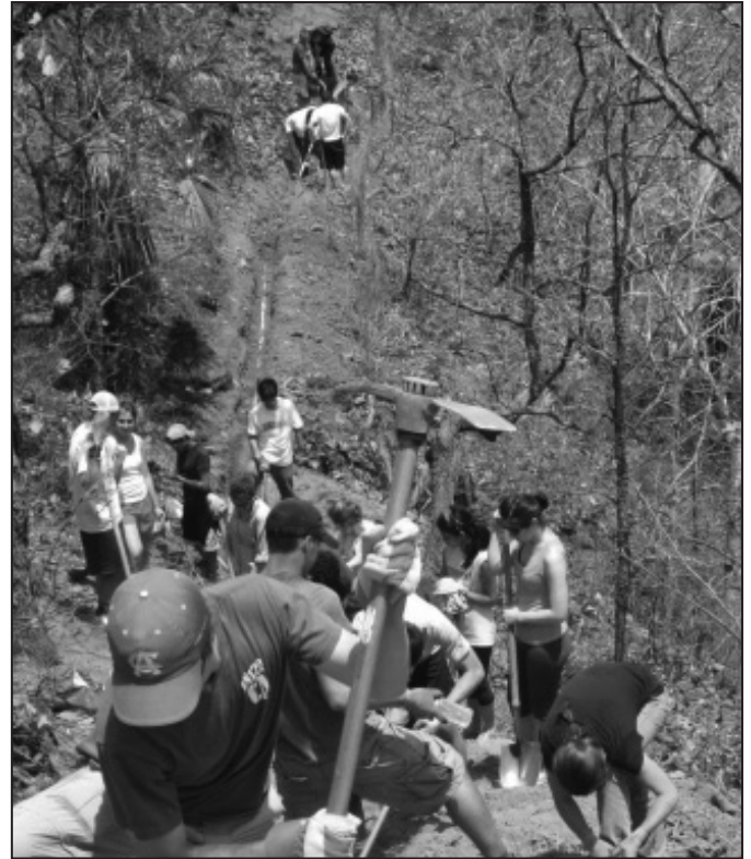
UA Global Water Brigade helps to install a pipeline in El Canton, Honduras. Photo: Global Water Brigades Arizona
