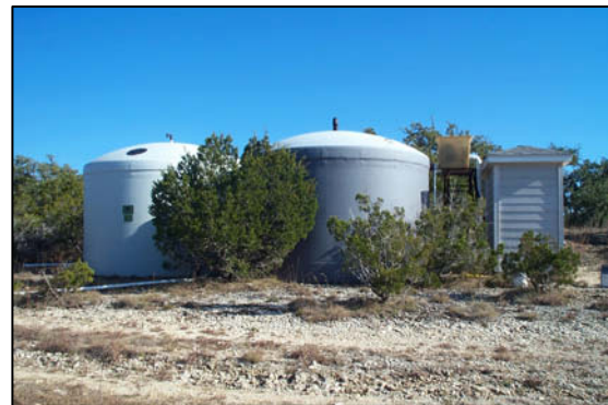
Figure 2-5. Two 10,000-gallon fiberglass tanks
