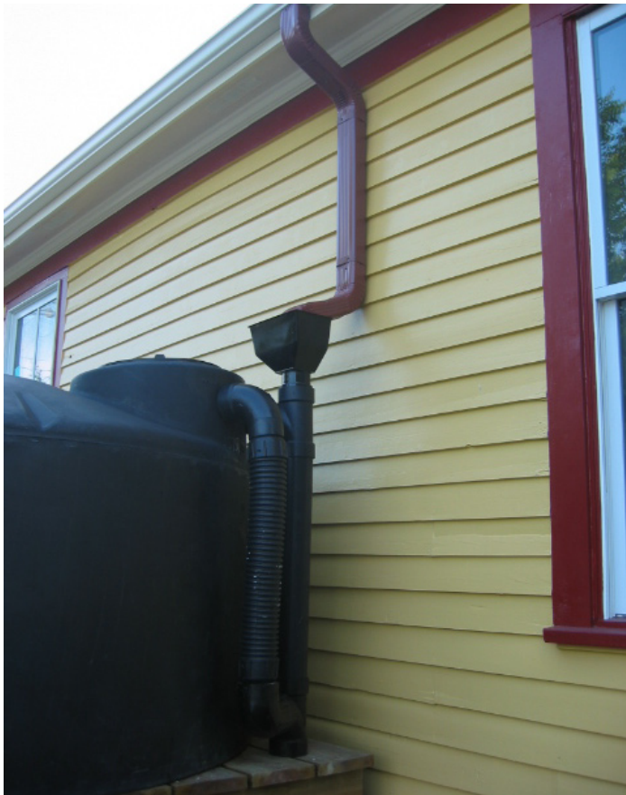
Figure 9. First flush diverter installed for a residential rainwater harvesting system
