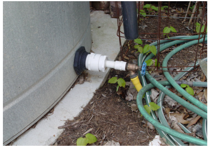
Figure 7. Bulkhead fitting installed at the base of a cistern
