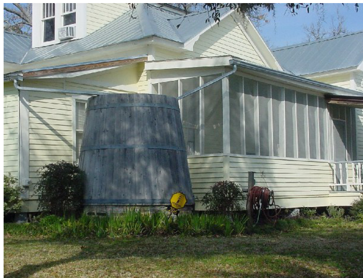
Figure 5. Above-ground cistern located at the corner of a house near existing downspouts (image courtesy of LSU Ag Center)
