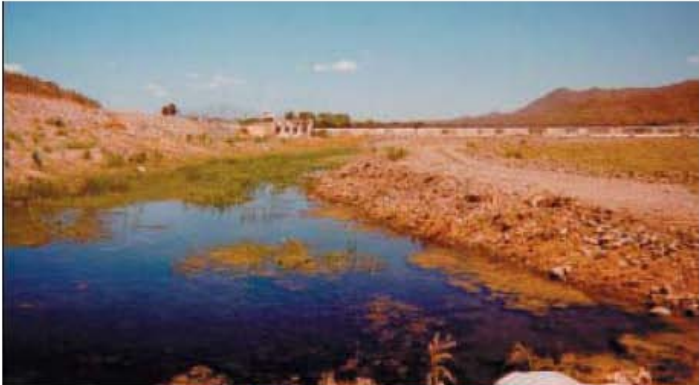
Water Seepage from Granite Reef Dam
