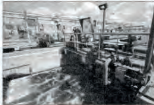
Wastewater treatment: Mechanic Phillip Castro does a routine inspection of the systems at a plant in San Antonio.
