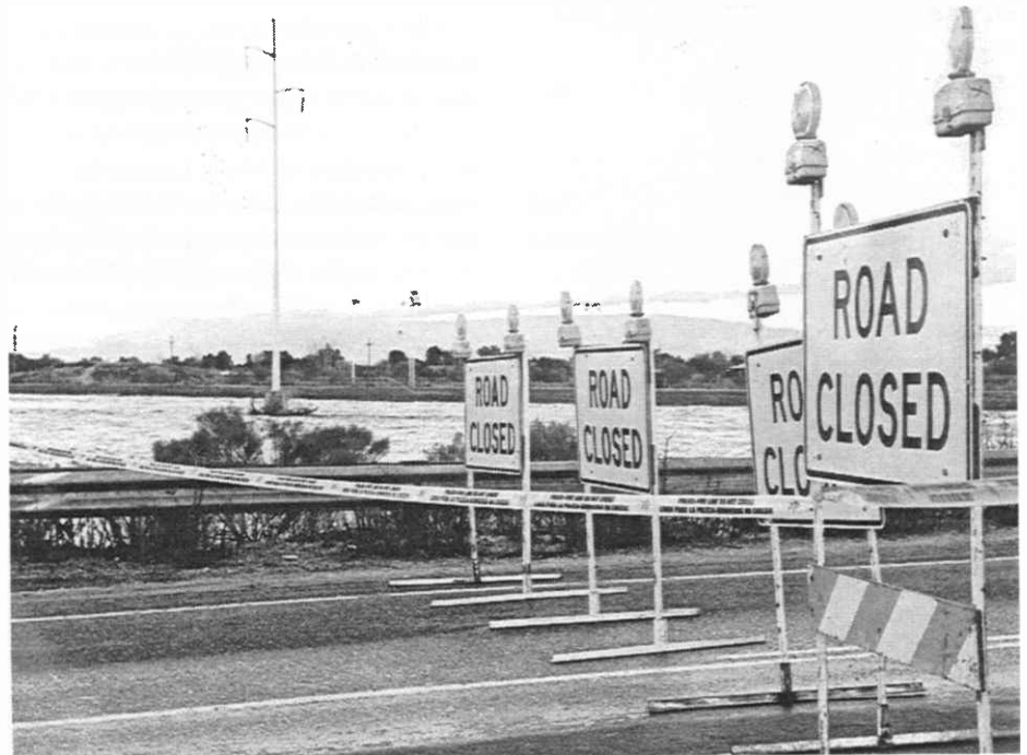
The bridge over the Rillito River at Dodge on the north side of Tucson typified dozens of crossings closed by high waters. While some embankments were damaged and approaches washed out, few bridges were destroyed, although several were damaged. (Photo: Barbara Tellman)
