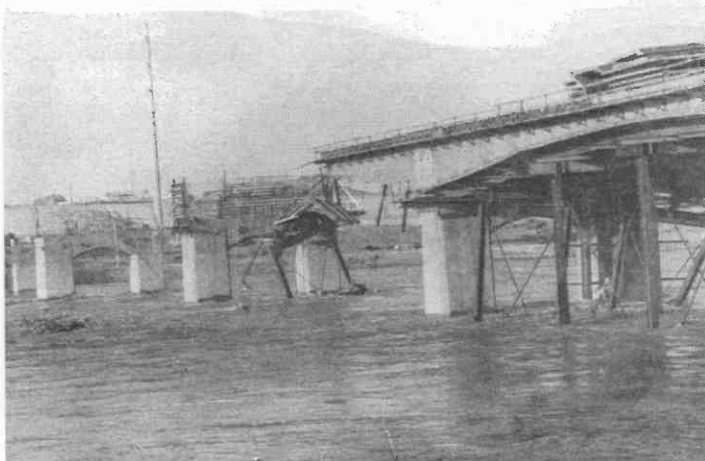
The new Tempe Bridge currently under construction over the Salt River suffered extensive damage. (Photo: Barbara Tellman)
