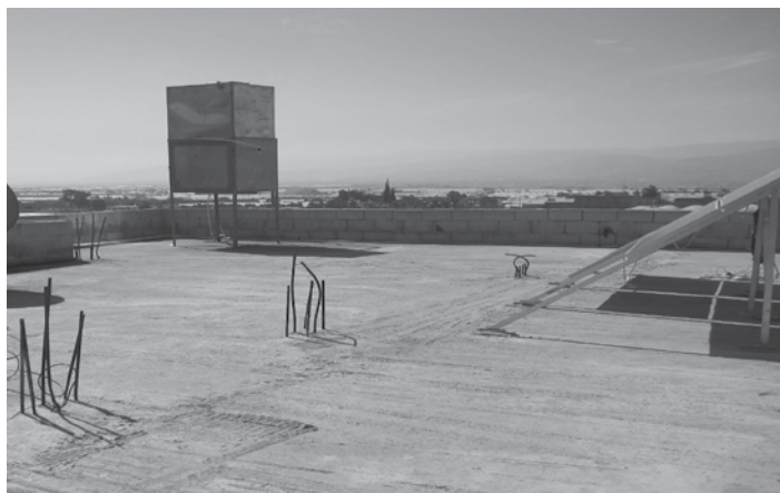
Rooftop tank and solar array for distribution of filtered gray water to plantings. Source: Sharon Megdal, WRRC
