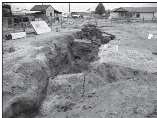
A fissure that opened unexpectedly near Queen Creek this summer. Photo: Arizona Geological Survey
