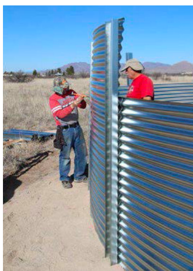
Figure 12. Bolting together a 28,000-gallon steel tank requires around 1,000 large nuts and bolts. A flexible monofilament, polyethylene liner fits inside the assembled tank. Photo courtesy of Oasis Water Harvesting.
