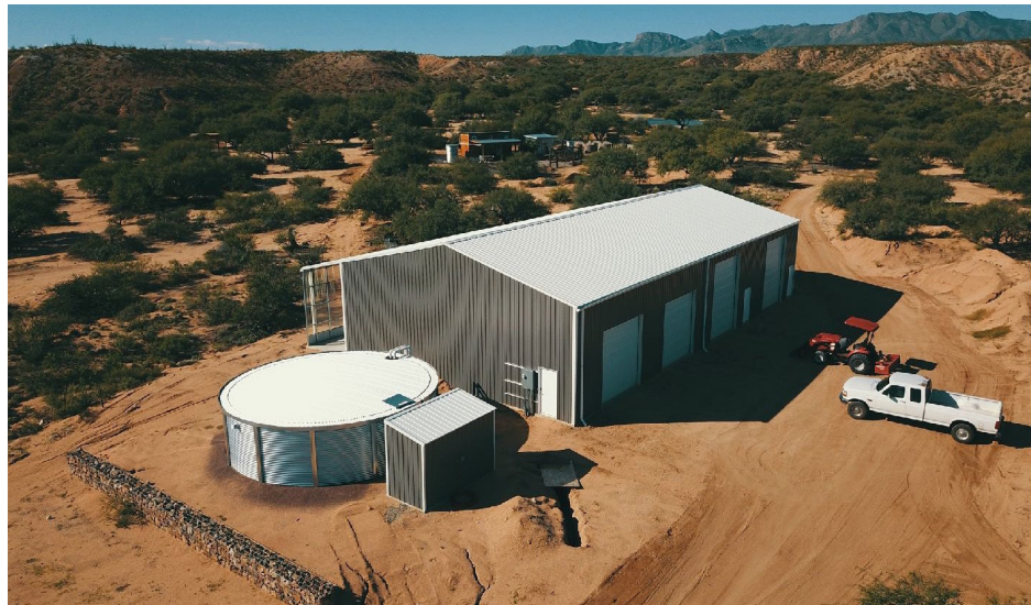
Figure 1. A circular cistern and pump-filtration shed store and process rain captured from a multi-use out building. St. David, Arizona. Photo courtesy of Derek 'Handeeman' Howlett.
