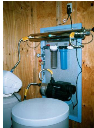
Figure 11. Typical treatment installation of an on-demand pump, 5-micron fiber filter, 3-micron activated charcoal filter, and an ultraviolet lamp (top). Photo courtesy of Texas AgriLife Extension Service.
