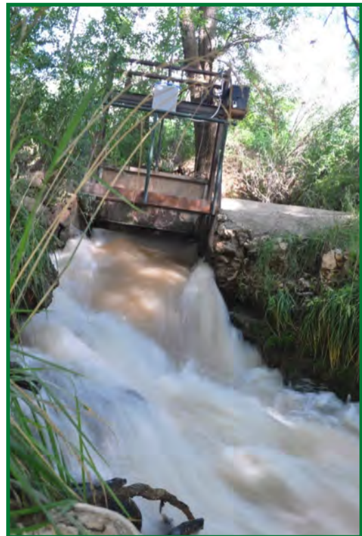
New automated ditch gate on the Vere River. Photo courtesy of Kim Schonek.
