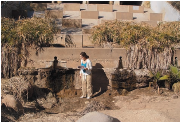
Brosnihan during field visits in 2009 to analyze scour issues in drainage ways in Green Valley, AZ.
